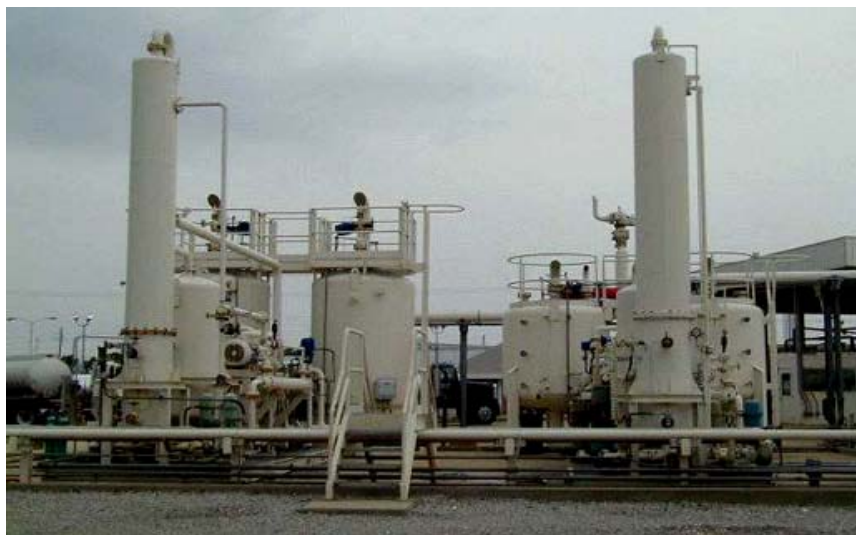
Figure 3 Example of Terminal Vapor Processing Unit
